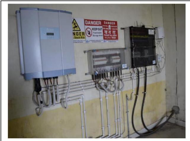
SOLAR CONTROL PANEL
